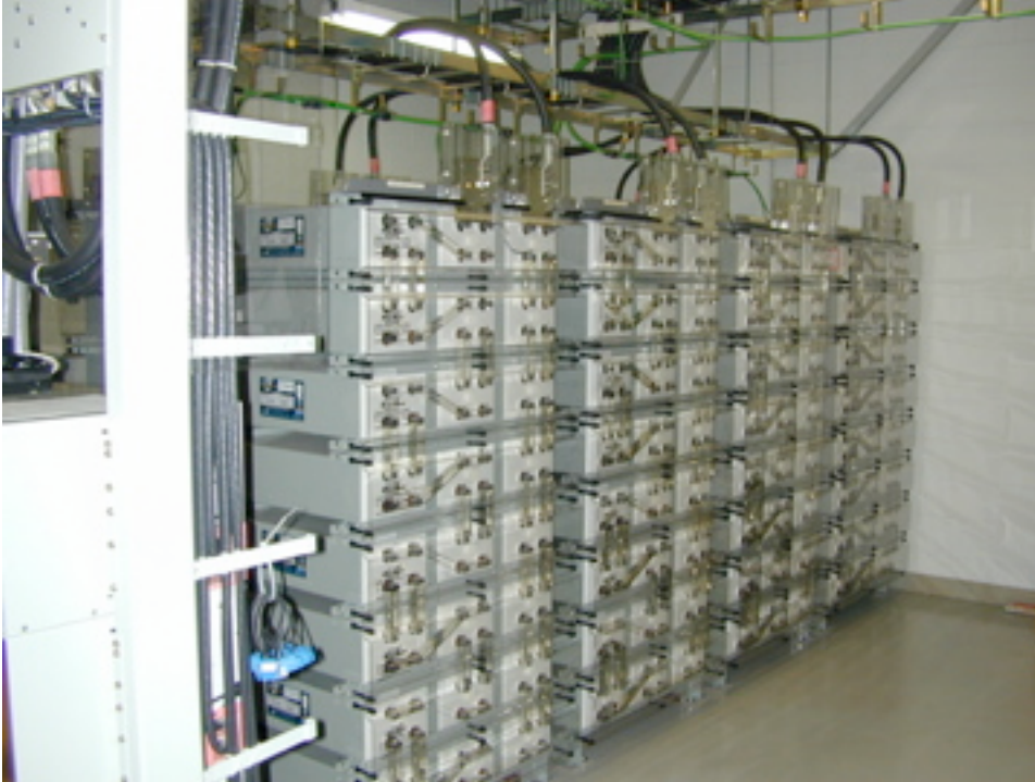
Figure 15. Nedonna Station, Battery Plant
