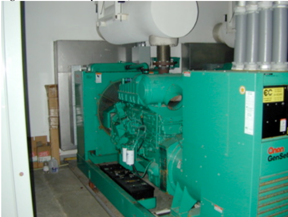
Figure 21. Pacific City Station, 2x300kW Generator Sets
