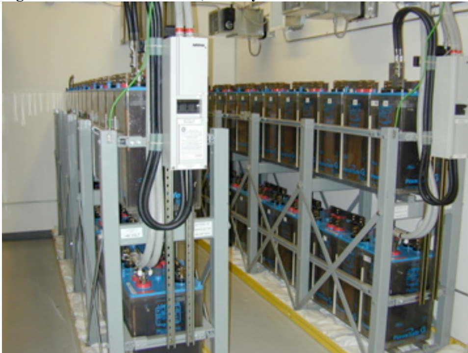
Figure 10. Warrenton Station, Battery Plant
