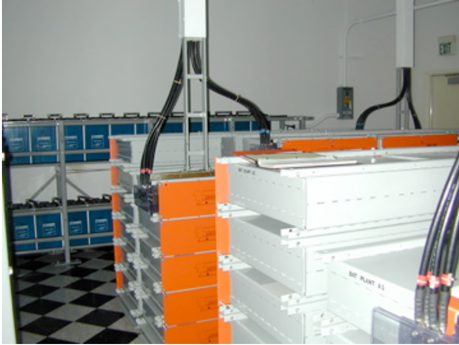
Figure 20. Pacific City Station, Battery Plant
