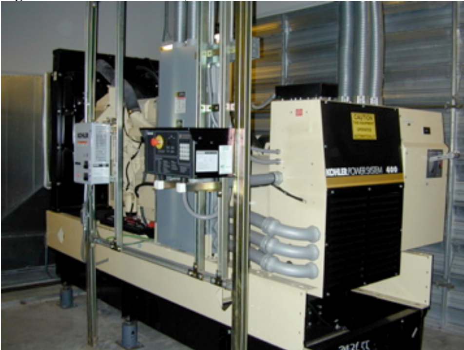
Figure 16. Nedonna Station, 2x450kW Generator Sets
